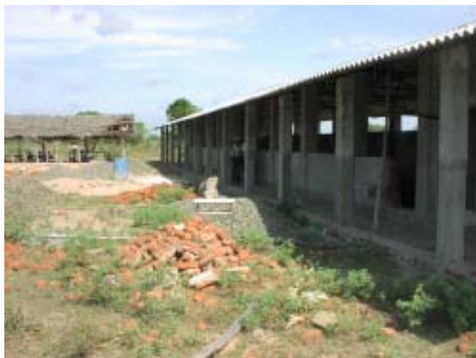
Primary school in Vaddavan, Eachchilampathai DS Division, temporary shed in the back and new school building under construction
